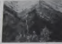
Fig. 106c. S. Stefano Romano. Foundation (part wall of ambulatory, right-hand wing) and I-pier.
